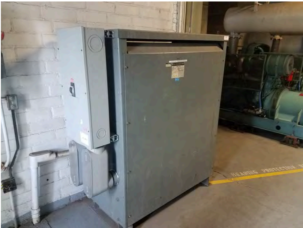
View of transformer in maintenance building.
